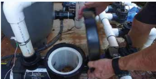
Circulation and filtration maintenance
